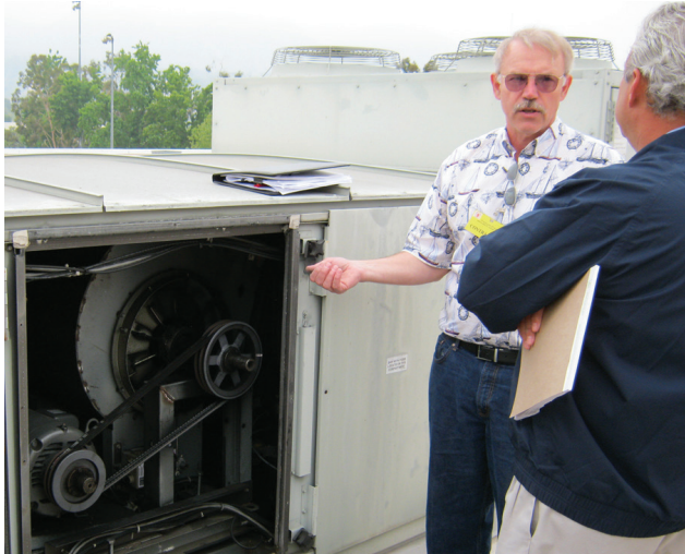
Site visit at a California MARFORRES facility.
