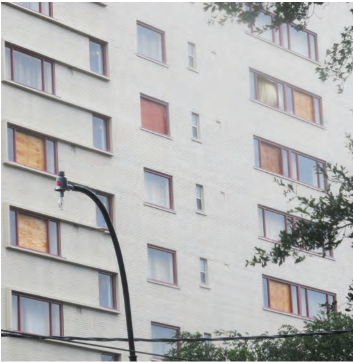
This image shows several boarded windows that were blown out by Hurricane Isaac in a hotel located adjacent to the Hotel Indigo.
