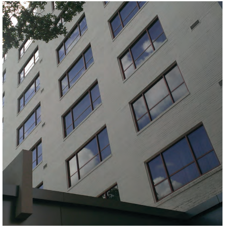
This image shows Hotel Indigo featuring Thermolite blast mitigation windows fully intact after Hurricane Isaac struck.
