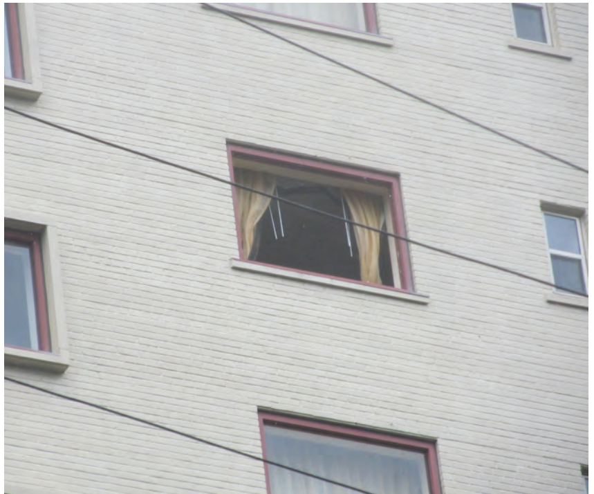
A closeup-view of a window in a New Orleans hotel that was completely blown out by Hurricane Isaac.
