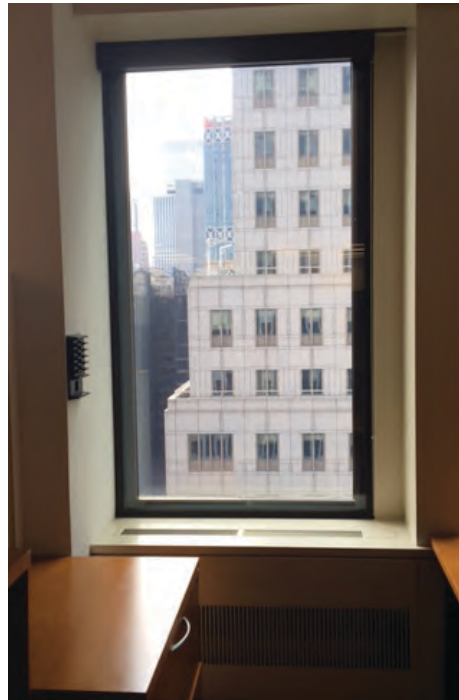
Thermolite's RetroWAL Gold fixed interior window system installed in one of the offices at the Jacob K. Javits Federal Office Building.
