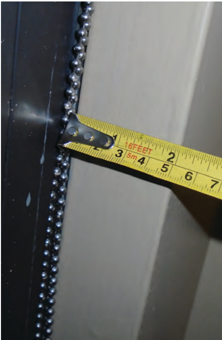
One of our installation technicians measures a two-inch wall pocket against the original window frame. Thermolite's RetroWAL system was installed on the opposite side of the gap, providing an effective thermal break.
